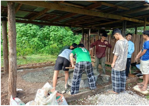
On 14 th August 2023, Students learn to work – building the pig cage under the supervision of Maitree.
